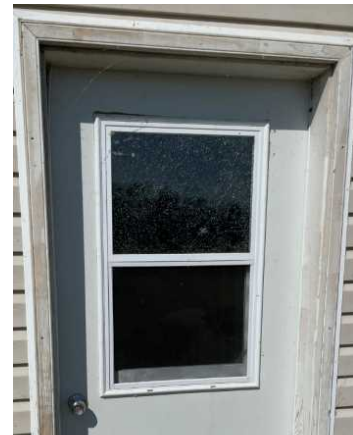
Garage door top window is rock chip shattered.
