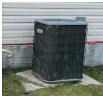
Central Air Conditioning
