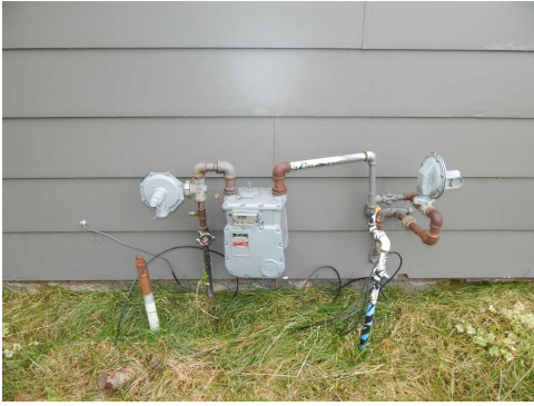
Gas meter at home meters gas used by both home and store
