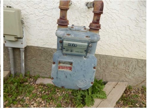
Located on west side of store - this meter is disconnected
