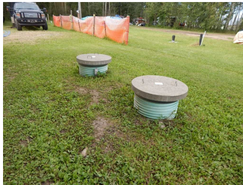
Sewer holding tanks for store
