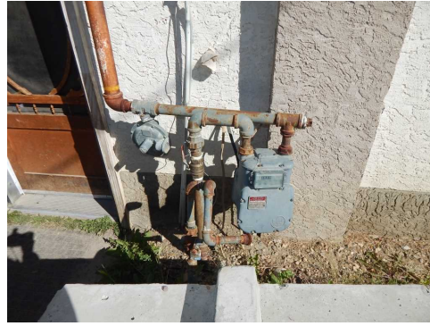
This does not meter the gas - it only is gas access to store.
