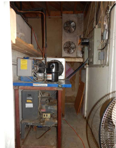
Compressor for cooler
