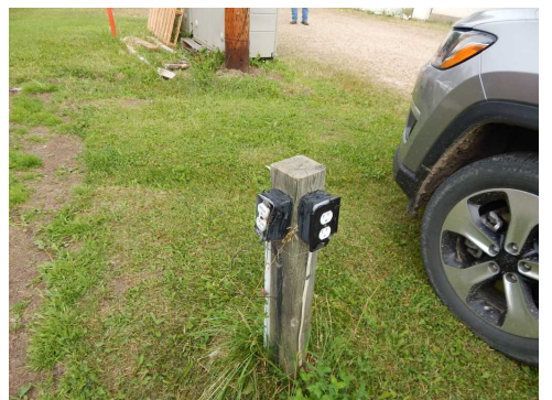
Power pedestal - not functional
