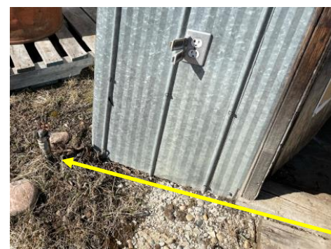
Water tap - summer use only located at SW corner of shop
