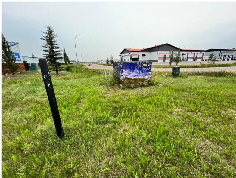
Photograph 8: Utility rough-ins, an electrical transformer and Telus pedestal located near the south boundary near McKenzie Crescent.
