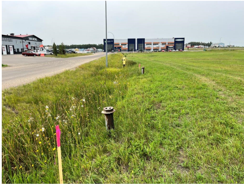
Photograph 9: Water utilities along the south portion of the Property and McKenzie Crescent.
