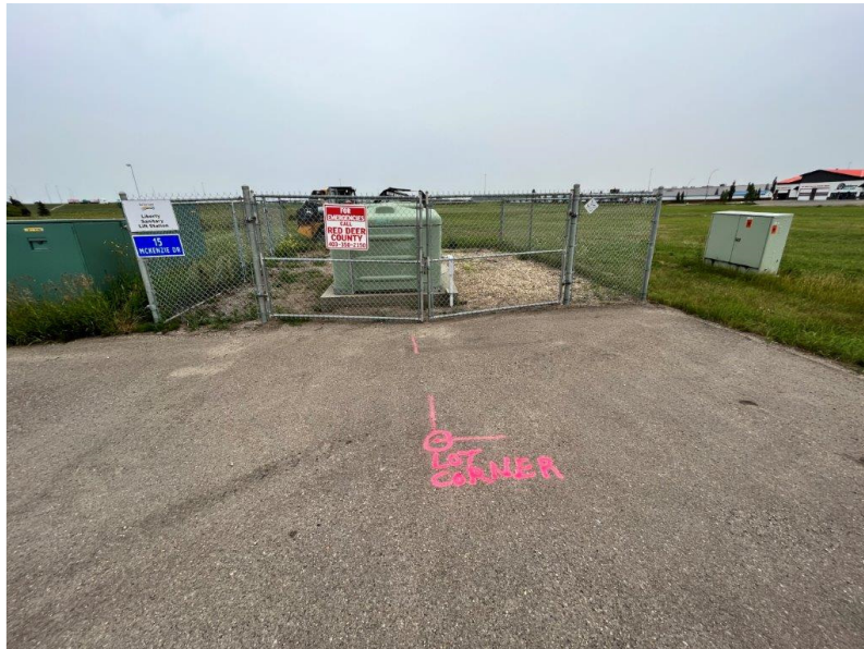
Photograph 12: The Liberty Sanitary Lift Station in the northwest portion of the Property.
