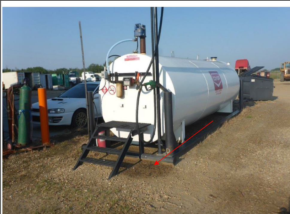
Photograph 14: This 13,000 L double-walled steel AST is located adjacent to the northwest corner of the Site and contains diesel fuel. An approximately 1 m 2 stain is visible near the fill point beside this AST.
