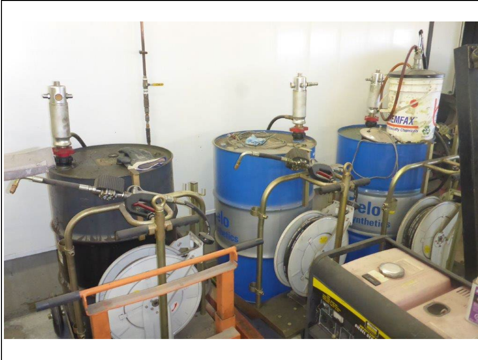
Photograph 11: Drums of lubricant used for servicing vehicles stored inside the shop.
