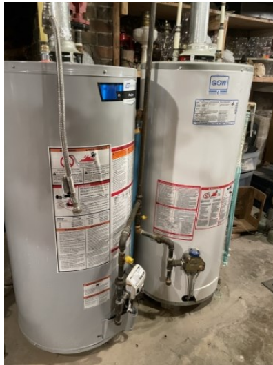
Grey HWT new in approximately 2018 services the radiant heat to the suite. The pump was replaced approximately 2-3 years ago.
