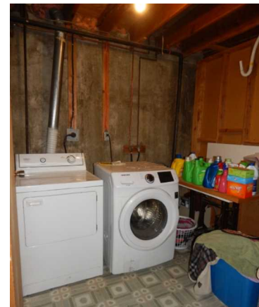
Laundry room in basement Washer & dryer are a couple of years old
