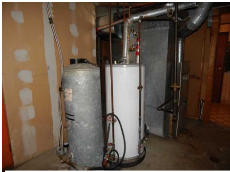
Utility room in basement
