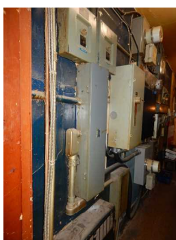
Electrical panel on main floor
