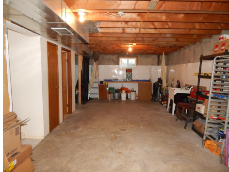
Interior weeping tile system has been installed around the entire basement - connected to sump located in utility room in south east corner of basement.
