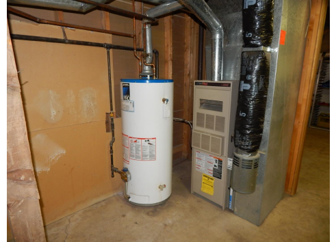
Furnace replaced in 2001. In past four years seller has replaced the motor of control module and last fall replaced the flame sensor.
