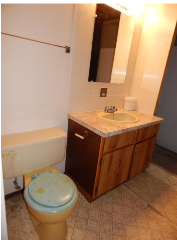
Sink is functional, but the toilet needs repair/replacement. Water has to be manually added to flush.
