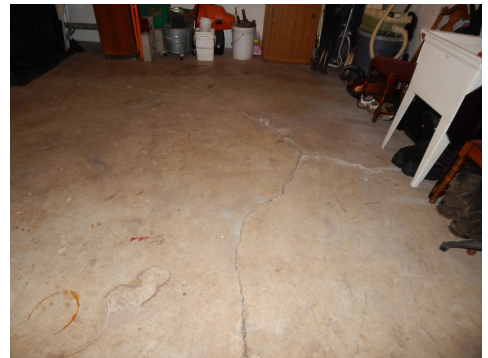
Basement floor of northwest portion of basement has a substantial heave. This heave has been there for long time.
