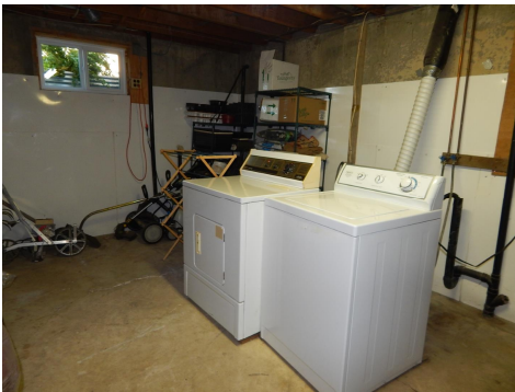
Washer & Dryer located in utility room in basement.
