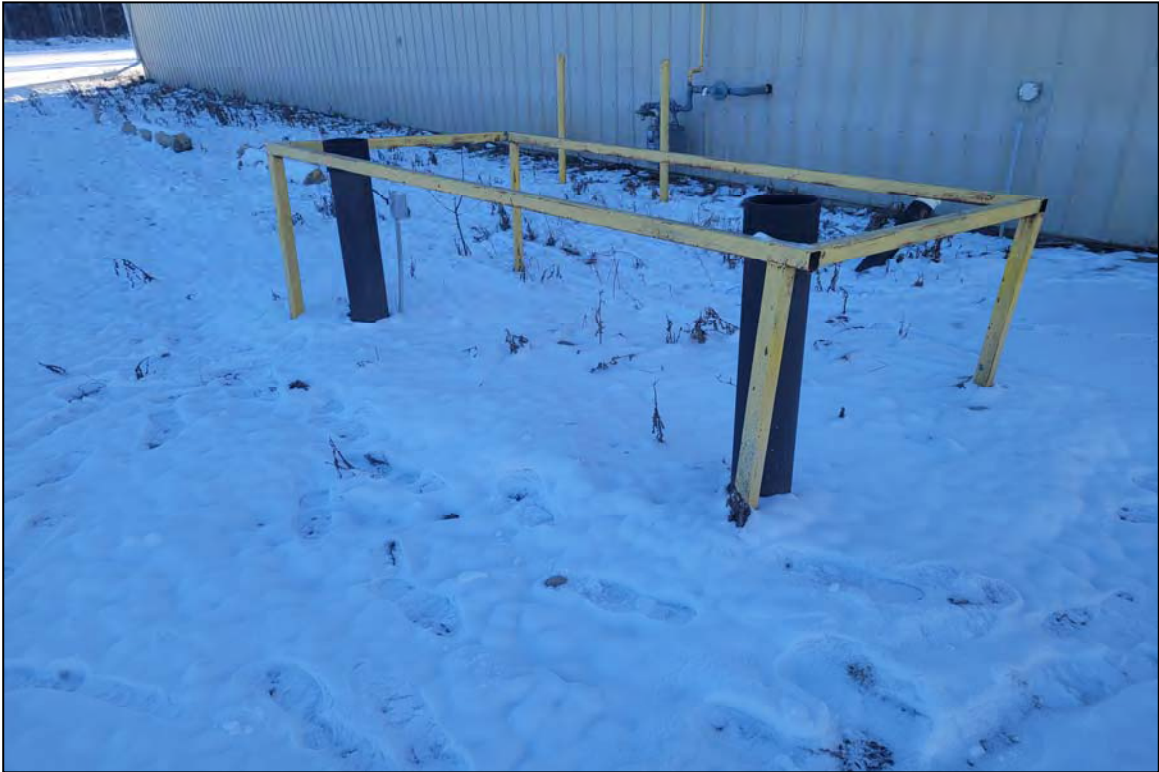
Photograph 9: Looking at septic system vents (Oct-25-23).
